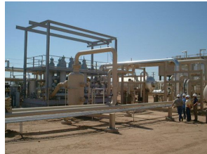
1 st gas processing
